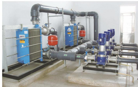
Plate Heat Exchanger & Pump Unit
